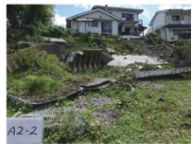
(i) L型擁壁の倒壊 (南阿蘇村)
