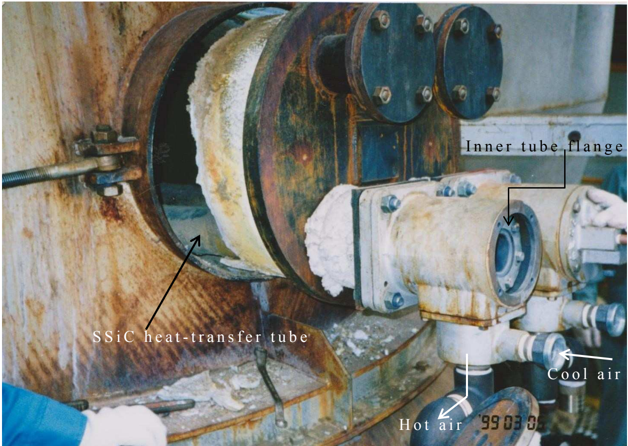
Fig.4.10 View of installed SSiC heat exchanger.
