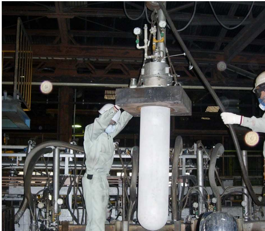
Fig.3.14 SSiC immersion tube with re-generated burner on the furnace of hot dip galvanized coatings.
