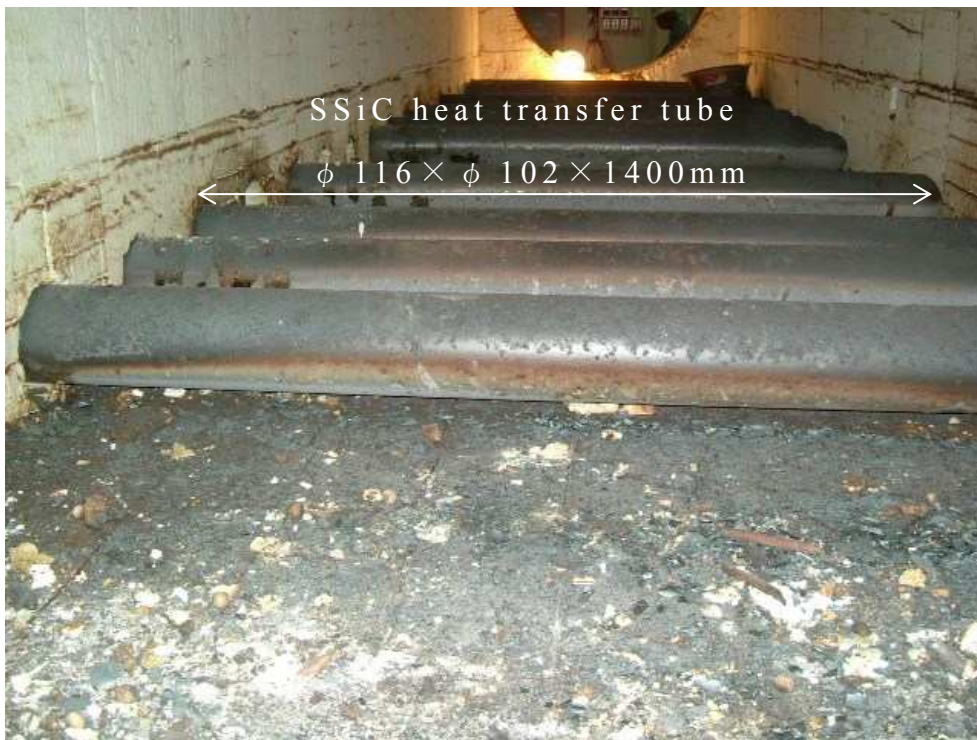
Fig.4.4 View of SSiC heat transfer tubes on high temperature furnace.
